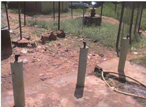
Plate 1: Dilapidated Pipe borne Water in Ankpa Urban
