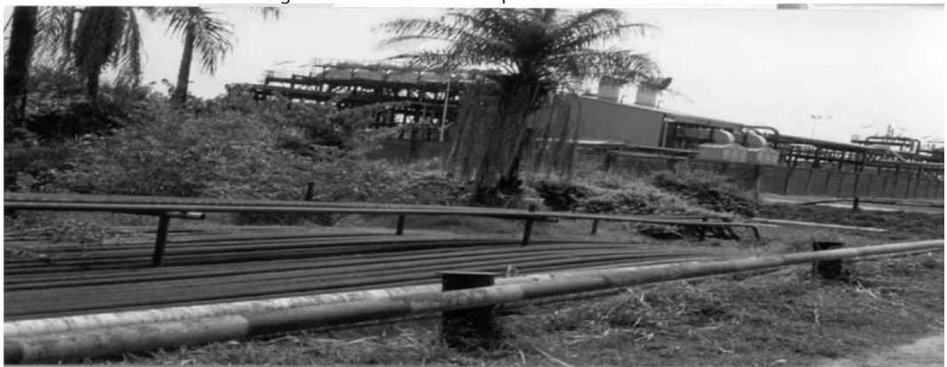
Surface Laid Rusted Oil Pipe Lines in Obagi
