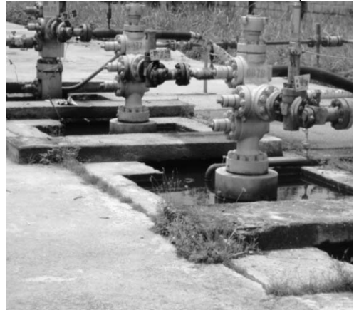
Open Oil Wells with Rusted Oil Well-Heads in Obite
