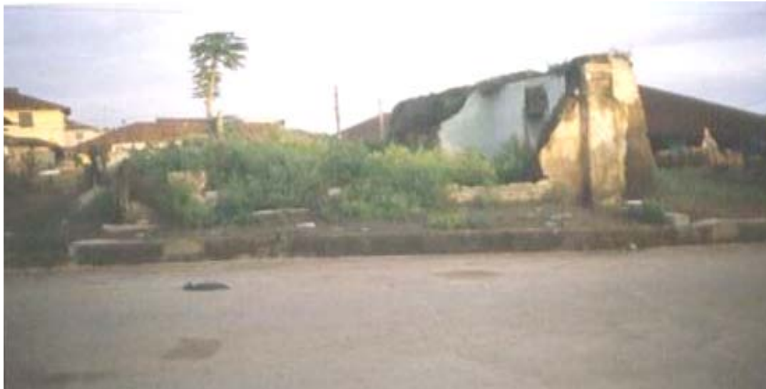
Plate 1b: Collapsed building left uncared for in the city core Source: Field Survey, 2010
