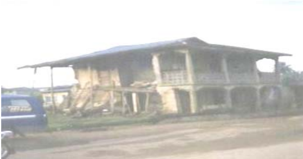
Plate 1a: Collapsed Buildings still inhabited by people due to high level of poverty Source: Field Survey, 2010
