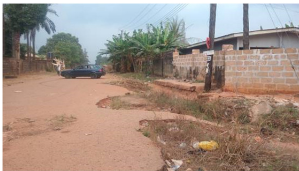
Plate 5. Showing the effect of erosion at EDPA Housing Estate, Ugbowo
