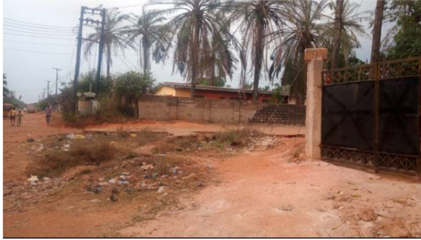
Plate 6. Showing the effect of erosion at EDPA Housing Estate, Ugbowo
